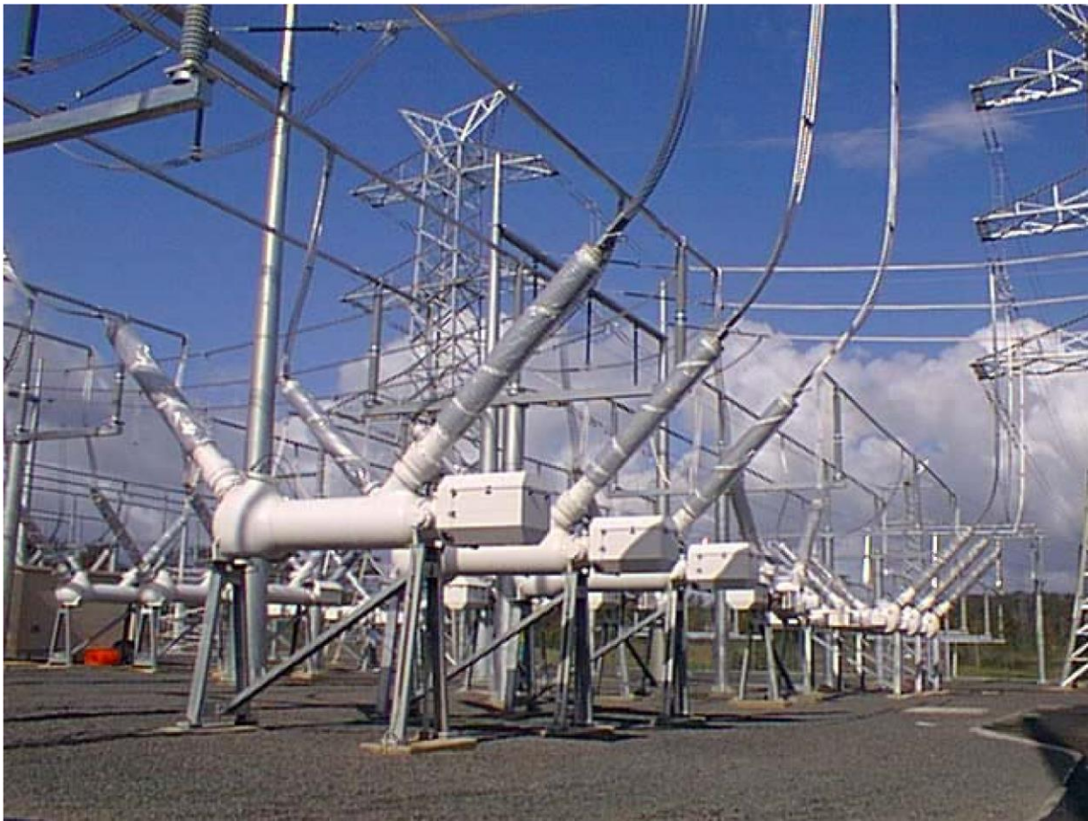
A view of an Electrical Substation
